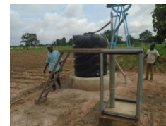
Rope pump water supply system for irrigation
